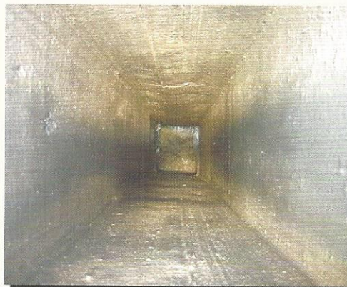
Fractured flue liners completely resurfaced.
