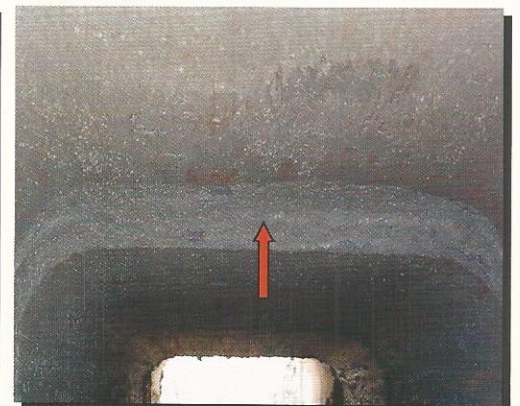
1" off-set between flue liners solidly filled.
