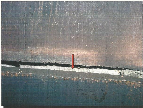
(2) Gap between flue liners as viewed through electronic scanner.
